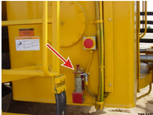
Hydraulic reservoir, right side
