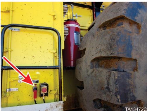
Electrical converter cabinet, left side
